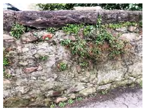
Further indication of plant growth that has penetrated the mortar joints in places
